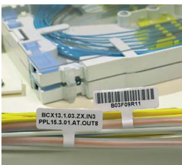
Fibre Optic Cable Markers
