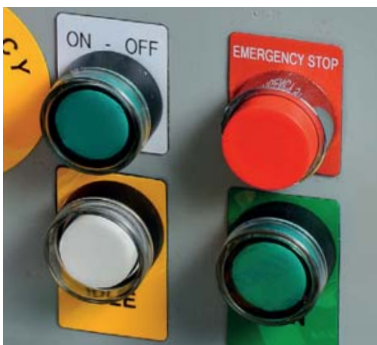
Control Panel Labels
