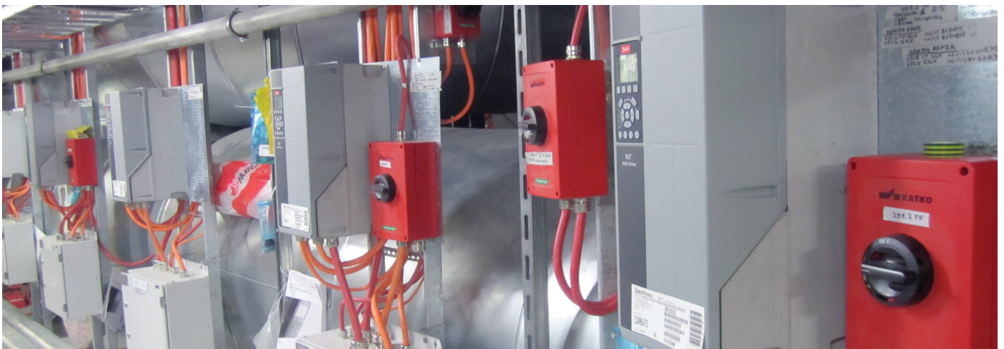
KEA Firerated safety switches installed at Keilaniemi metro station in Espoo, Finland
