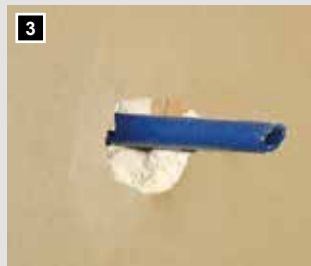
3 The dry wall builder knocks out a hole with a hammer and lets the central spike get through, this serves as a centre for the drill bit.
